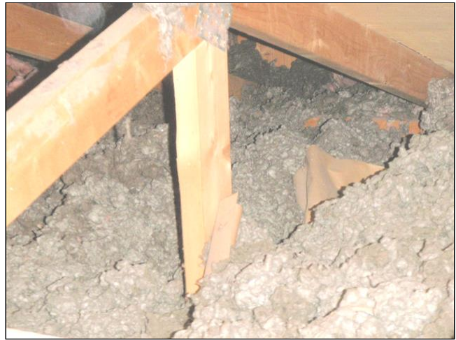
5.3 INSULATION Item 1(Picture)
