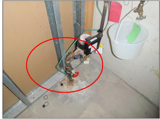
14.1 MAIN WATER SHUT-OFF Item 1(Picture)
