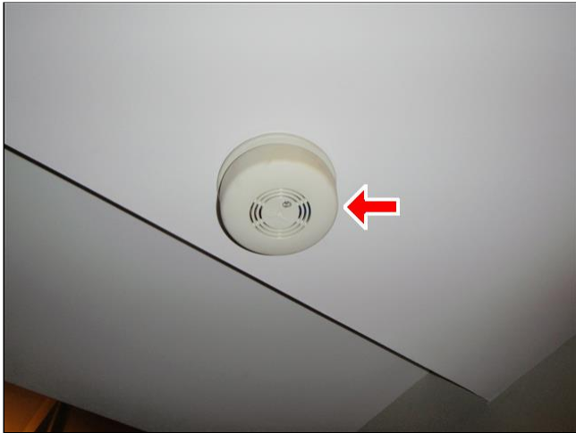
8.8 SMOKE DETECTOR TEST Item 2(Picture)
