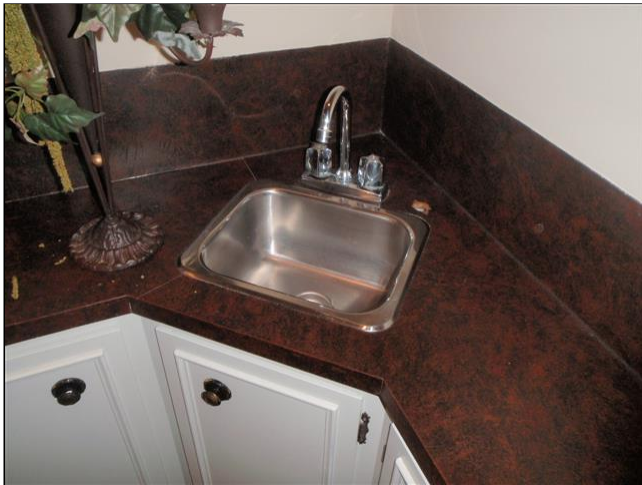
7.0 PLUMBING / SINK Item 1(Picture)
