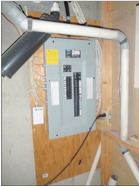
12.3 DISTRIBUTION PANEL Item 1(Picture)
