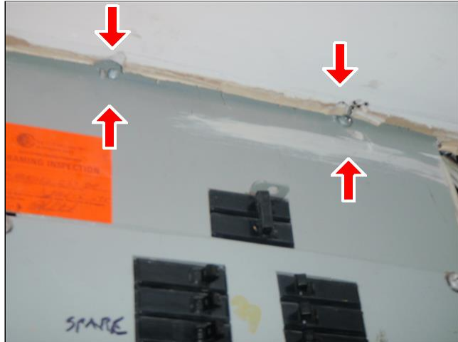
12.4 SUBPANEL(S) Item 1(Picture)
