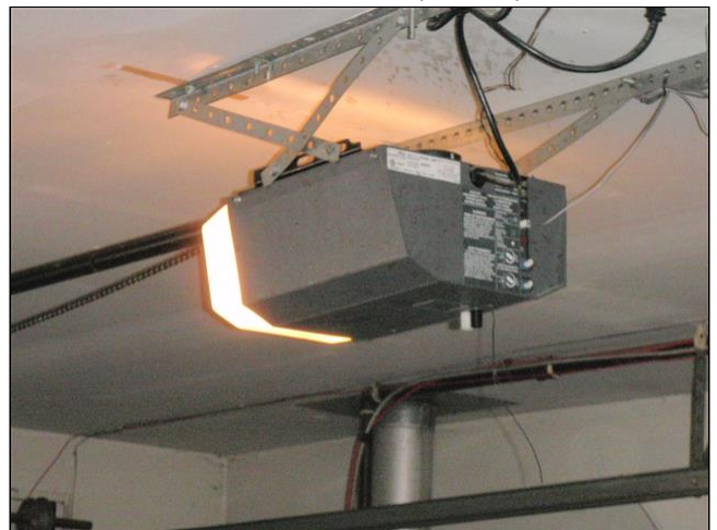
4.10 DOOR OPERATOR(S) Item 1(Picture)
