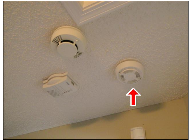
8.8 SMOKE DETECTOR TEST Item 1(Picture)
